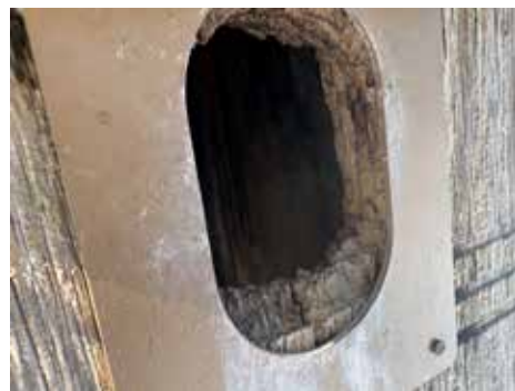
Use a protector plate to cover entrance hole and prevent further damage. (Steve Fallon)
