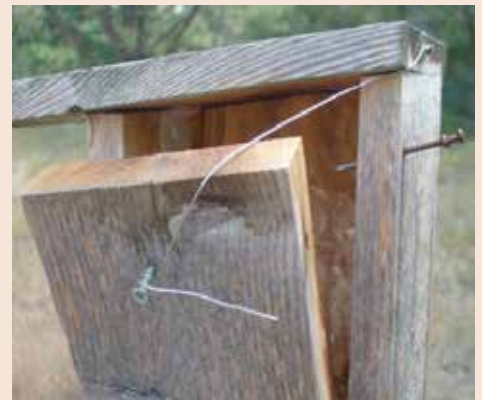
Wiring boxes open to prevent woodpecker damage.
